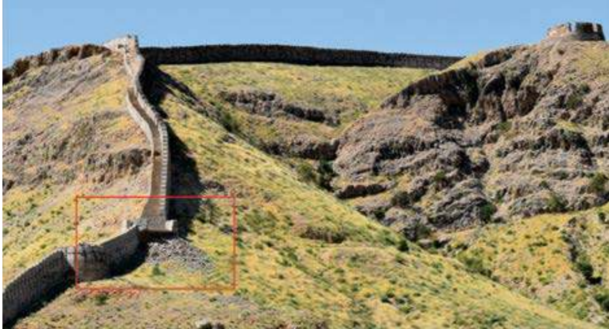
Collapsed bastion at Sann Gate, Ranikot
