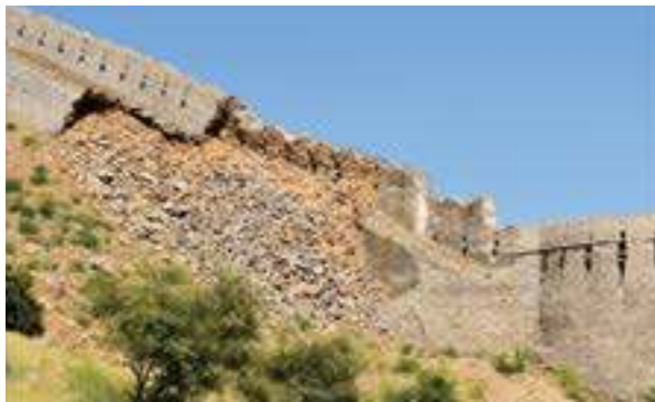
Rain damage at Sunn Gate, Ranikot
