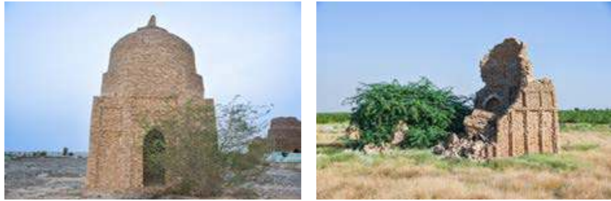
Tomb collapse in Aararo Makam, Dadu
